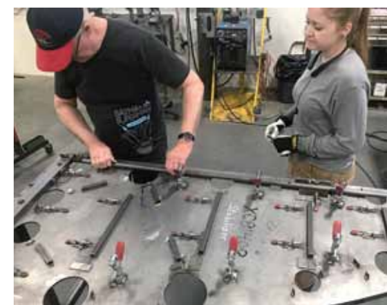
From top: Bending the rudder with Mark; trimming steel for the stabiliser; Pattie the welder supervising. Next page: second visit.
