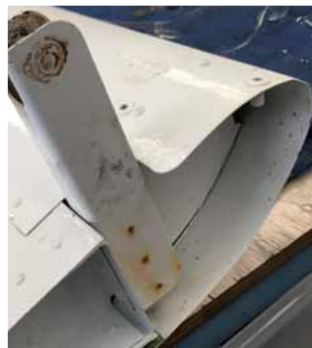
Not easy to see in this photo, but with flaps removed, evidence of corrosion on the nose riblet was easy to see in the paint.
